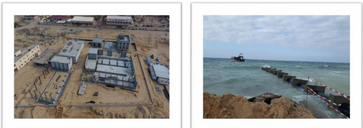
Figure 16: Gaza STLV Desalination plant
