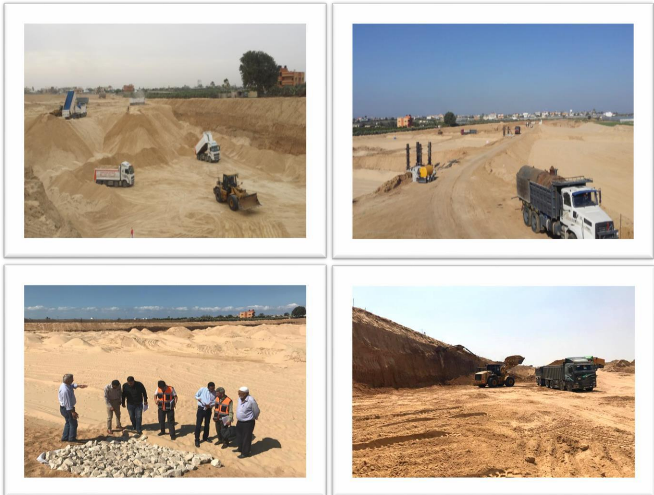
Figure 27: Infiltration Basin at Al Fokhari
