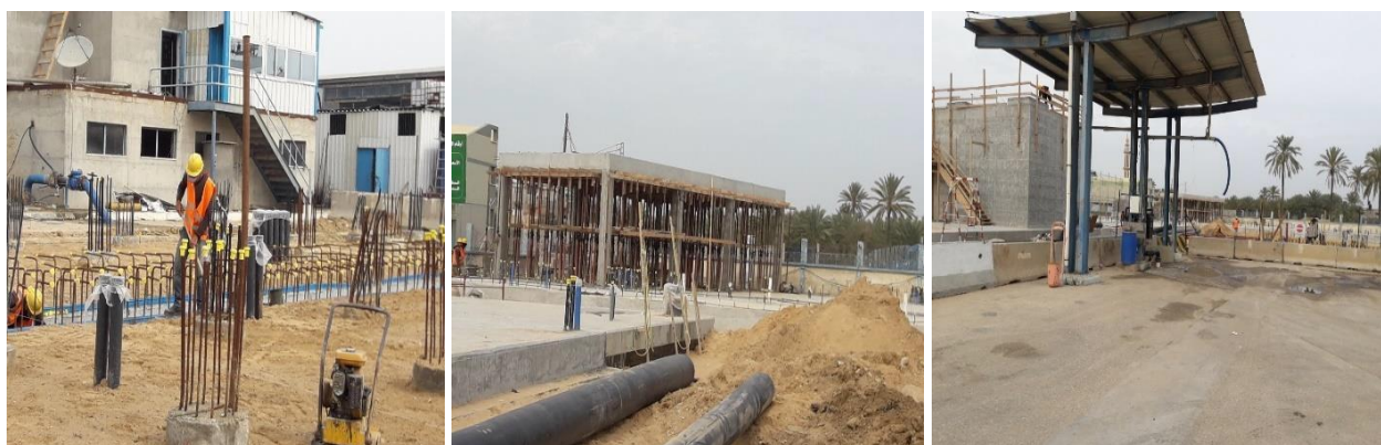
Figure 13: Deir Al Balah Sea Water Desalination Plant
