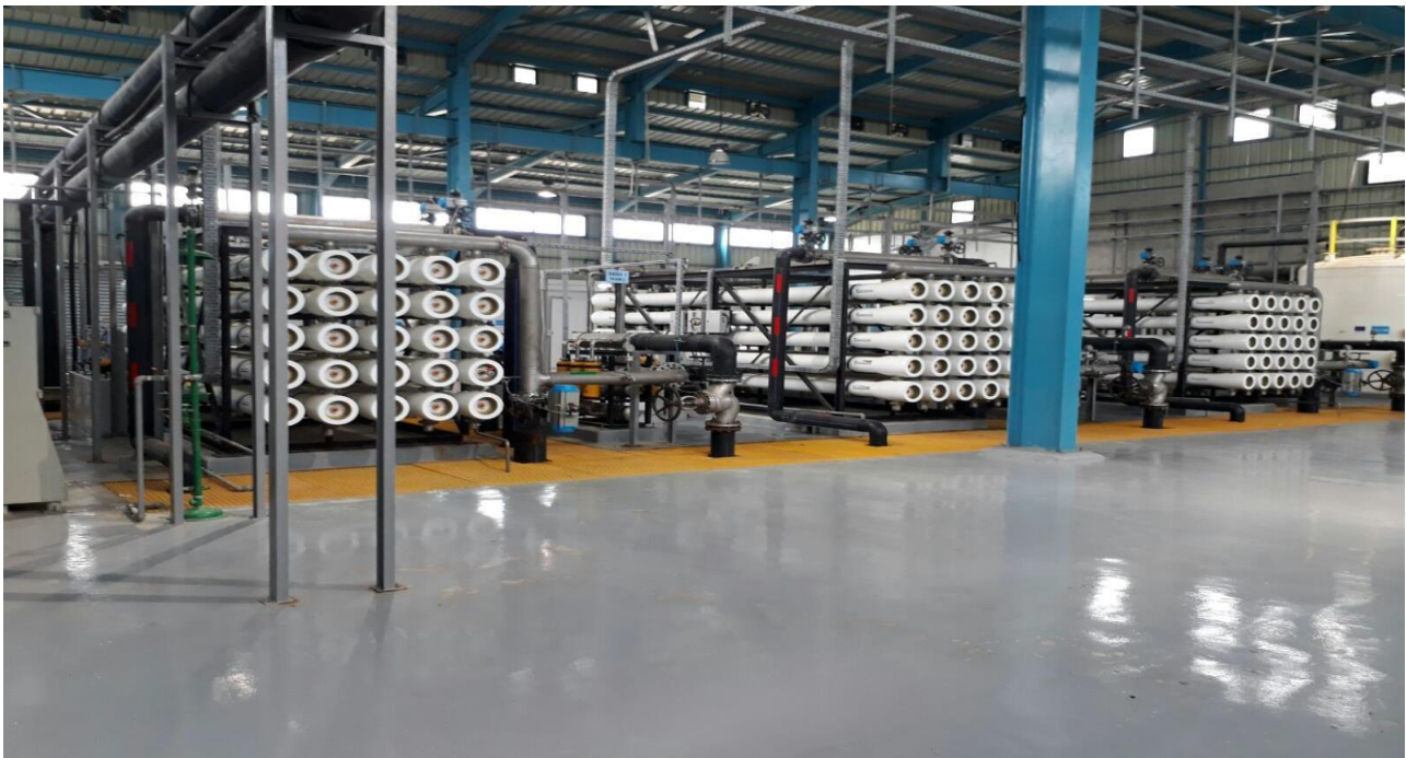
Figure 14: Sea Water Desalination Plant – Southern Governorates
