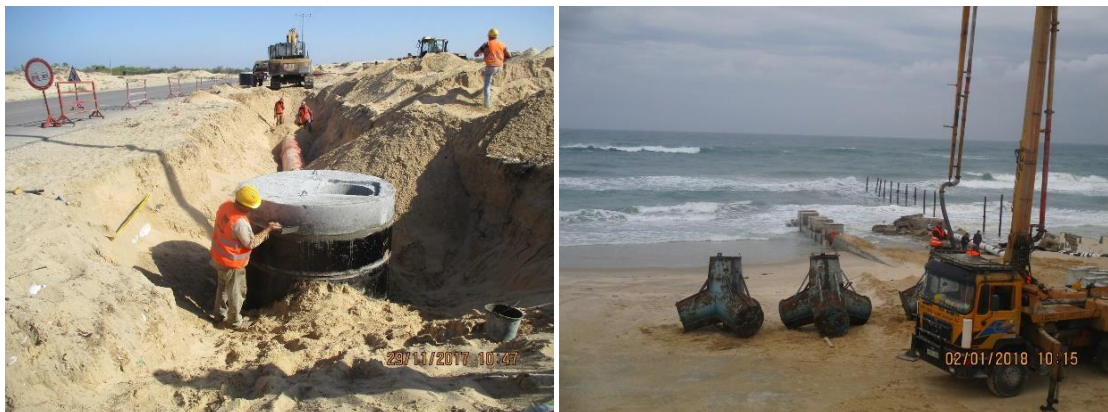
Figure 21: Effluent pipeline to the sea
