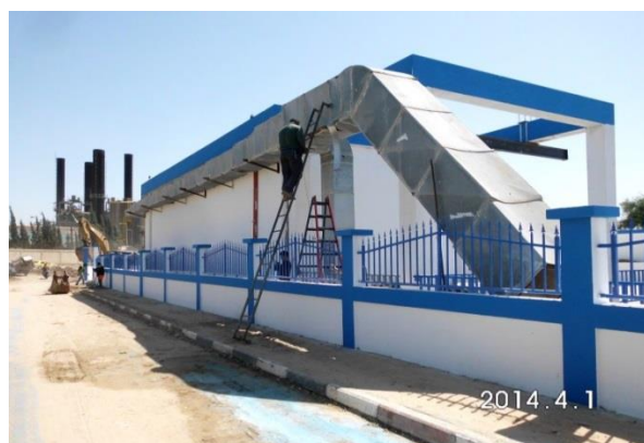
Figure 30: Al Nussirat Sewage Pumping Station
