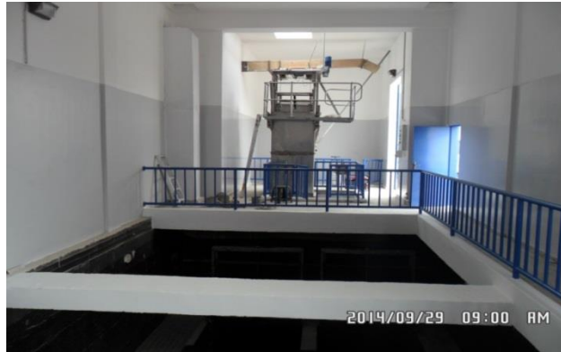
Figure 33: Al Nussirat Sewage Pumping Station
