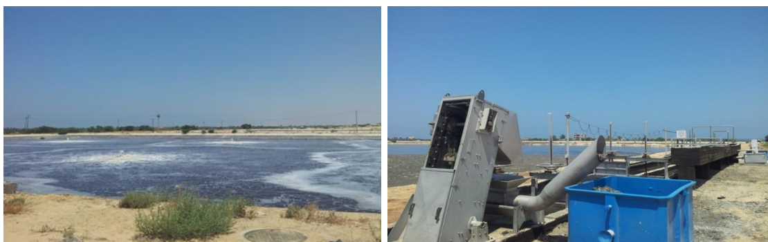
Figure 28: Khanyounis Temporary Wastewater Treatment Plant
