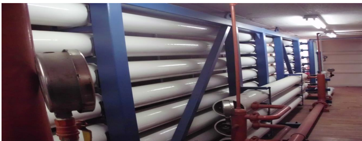
Figure 15: Water Desalination Works
