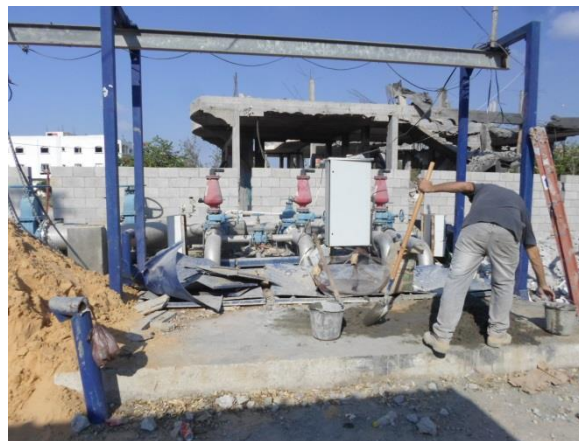
Figure 36: Beit Hanoun sewage pump station partially damaged
