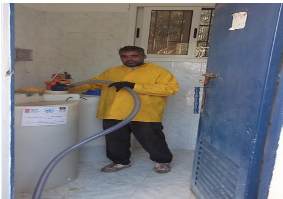
Figure 11: Chlorine Dosing Unit &amp; Chlorine filling in water well
