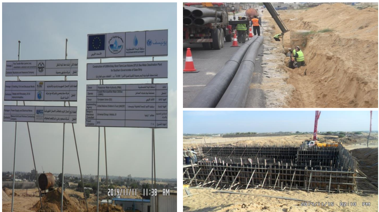
Figure 16: Sea Water Desalination Plant – Southern Governorates
