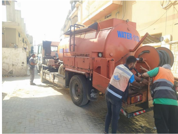
Supply and Install jetting pump for Nusirate Jetter
