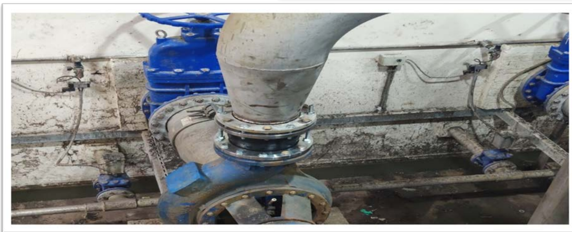
Figure 24 BLWWTP terminal pumping station Spare parts and maintenance activities
