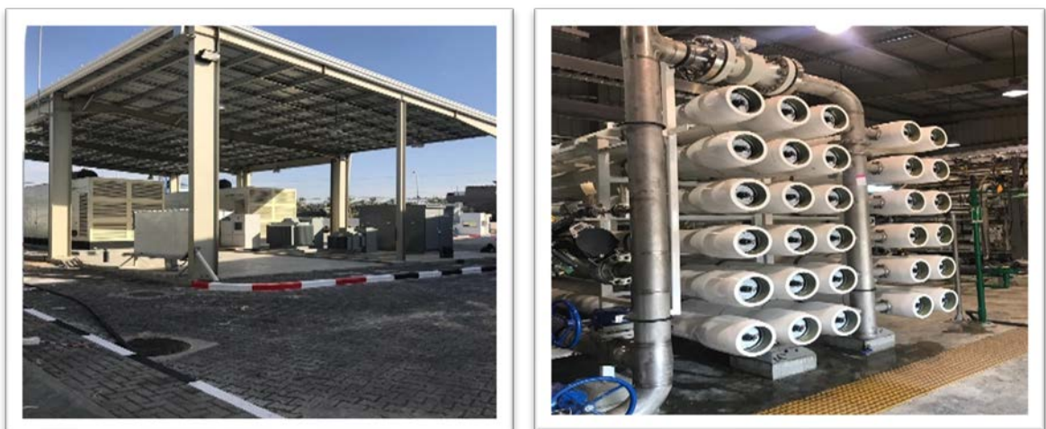
Figure 16 Deir Al Balah Sea Water Desalination Plant
