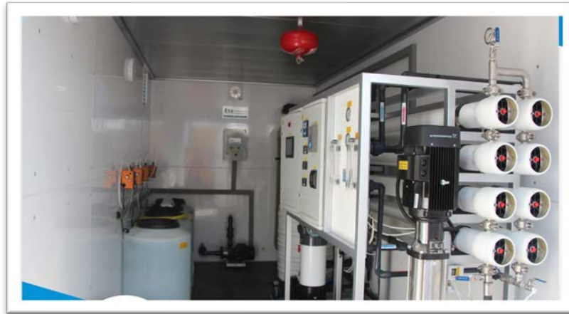
Figure 21 Abasan Al Kabera RO plant
