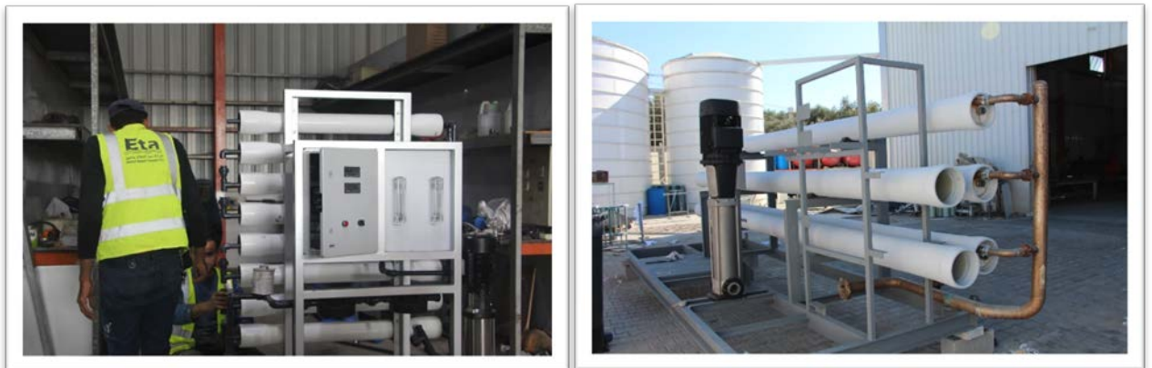
Figure 20 Rehabilitation of brackish RO plants
