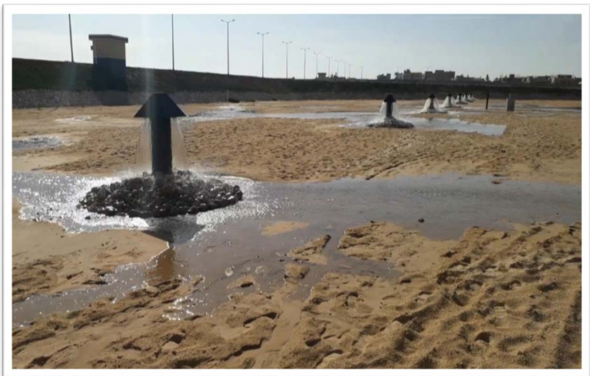
Figure 32 Infiltration Basin at Al Fokhari
