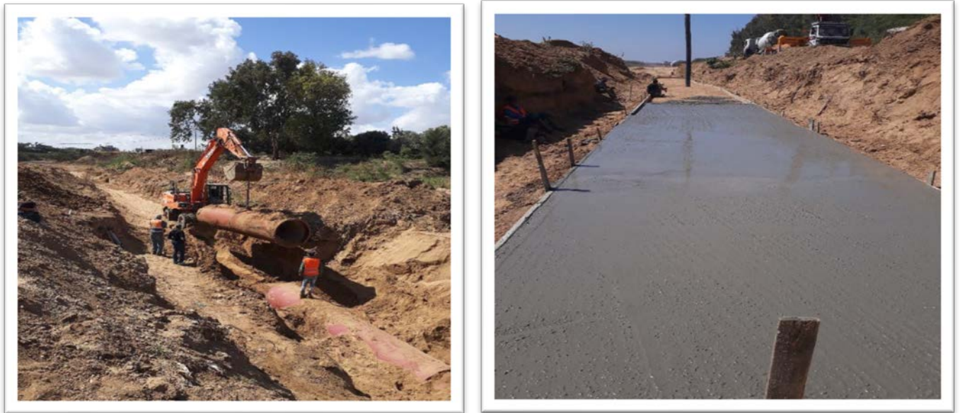
Figure 26 Central WWTP Pressure line
