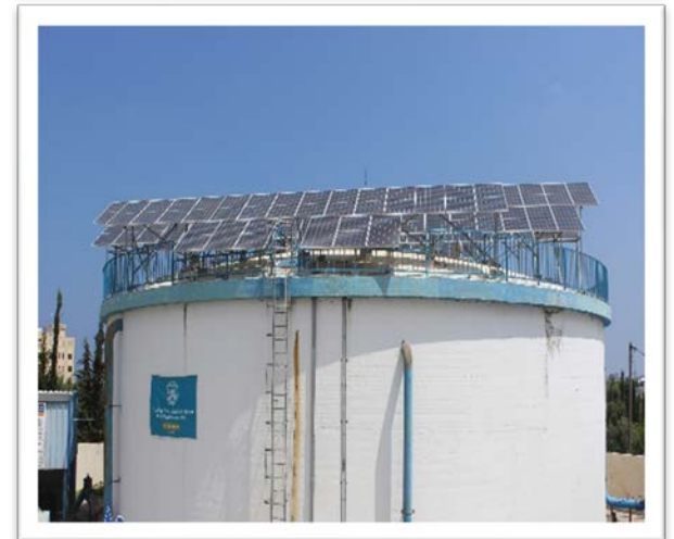
Figure 10 PV systems installed
