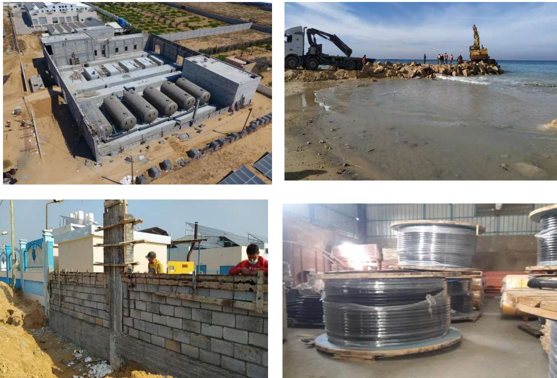
Figure 23 Expansion of Sea Water Desalination Plant – Southern Governorates
