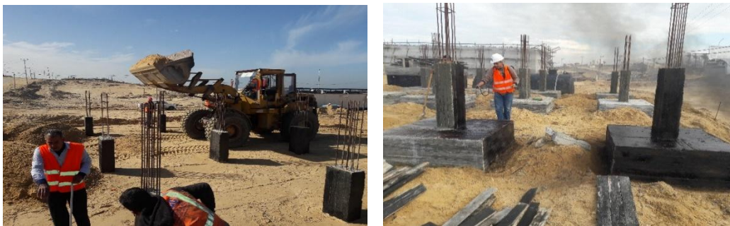
Figure 19: Gaza STLV Desalination plant
