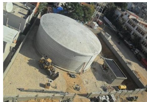
Figure 26: Civil Defense Water Tank
