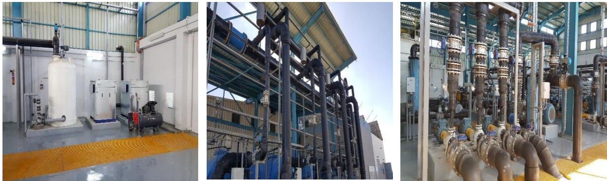
Figure 16: Sea Water Desalination Plant – Southern Governorates
