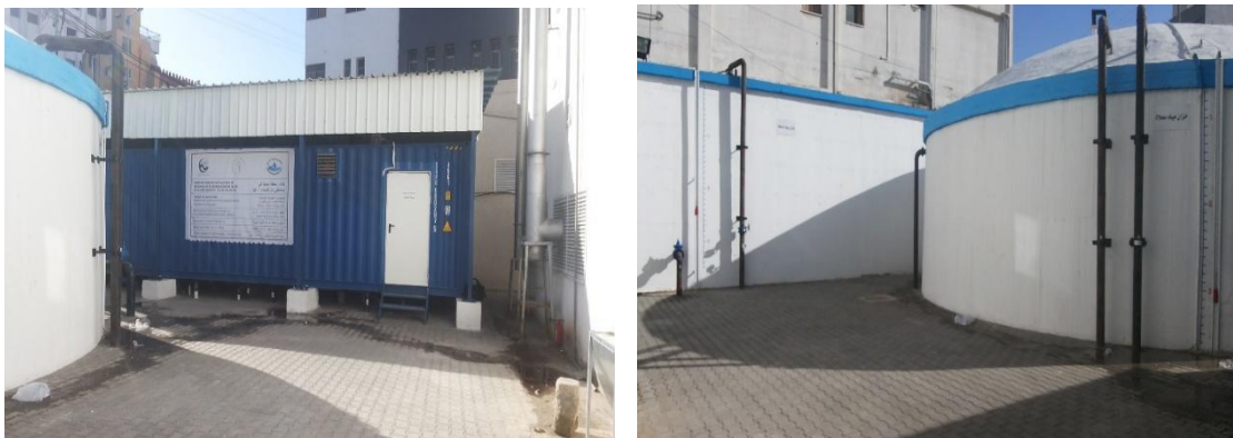
Figure 20: Containerized 500m 3 /day desalination plant
