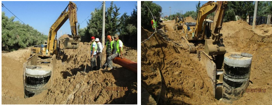
Figure 36: Wastewater Networks at Rafah & Khanyounis
