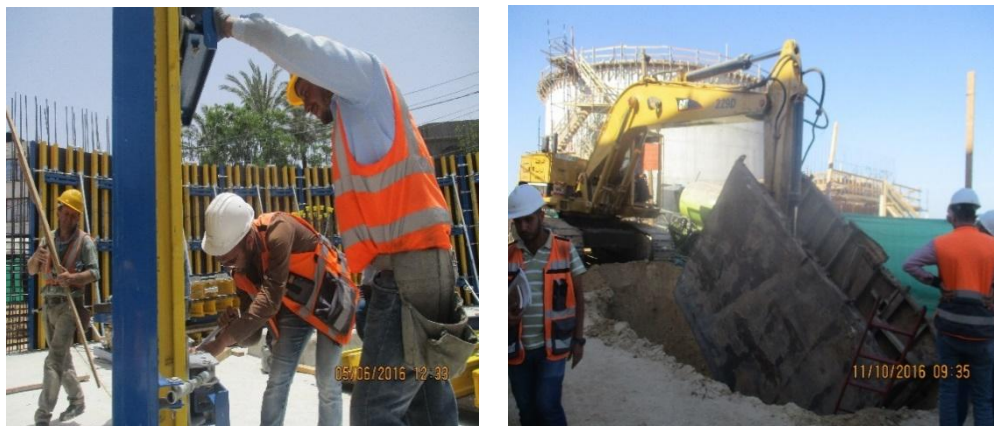
Figure 23: Beit lahia water tank
