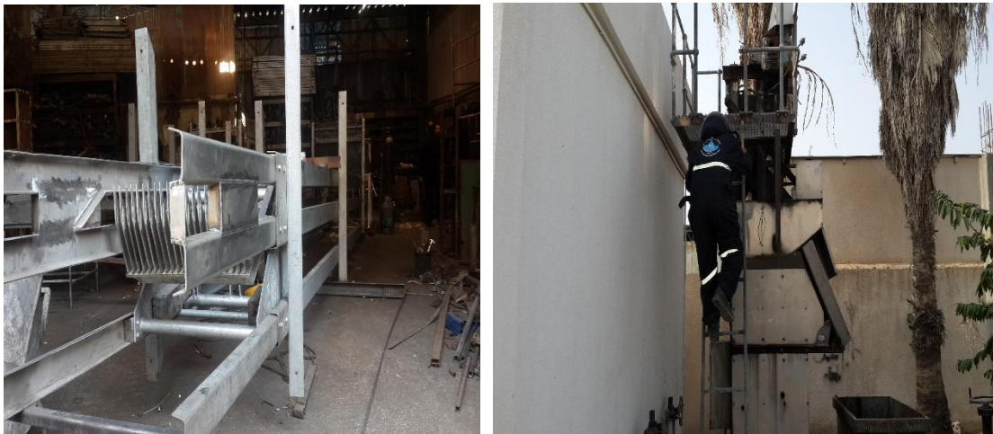
Figure 42 : Bar screen Maintenance
