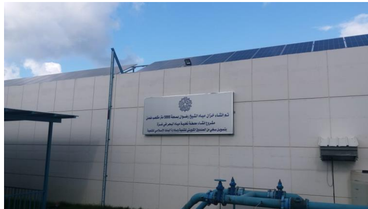
Figure 10 PV systems installed
