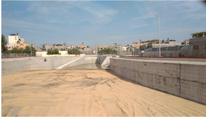
Figure 43: Aslan stormwater infiltration basin-Beit Lahia
