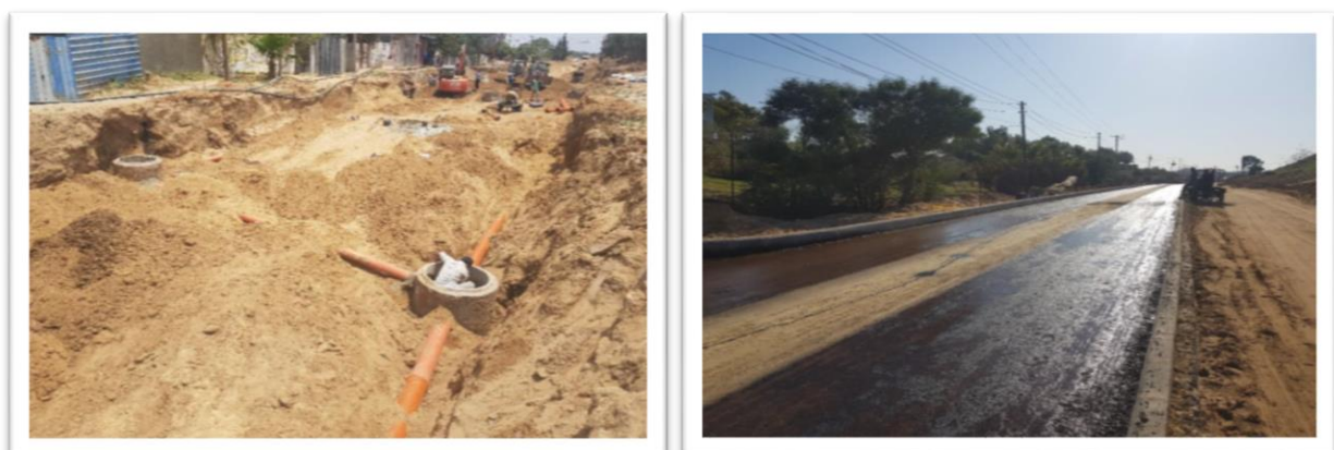
Figure 35 Central WWTP Gravity Pipeline
