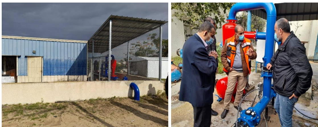
Figure15 Beit Hanoun water well
