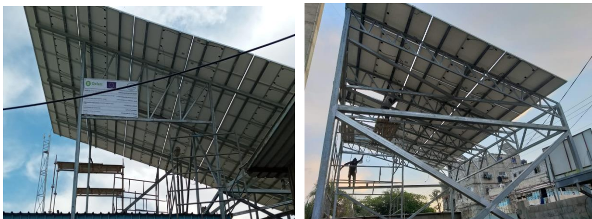
Figure 27 providing 6 RO plants with PV solar energy
