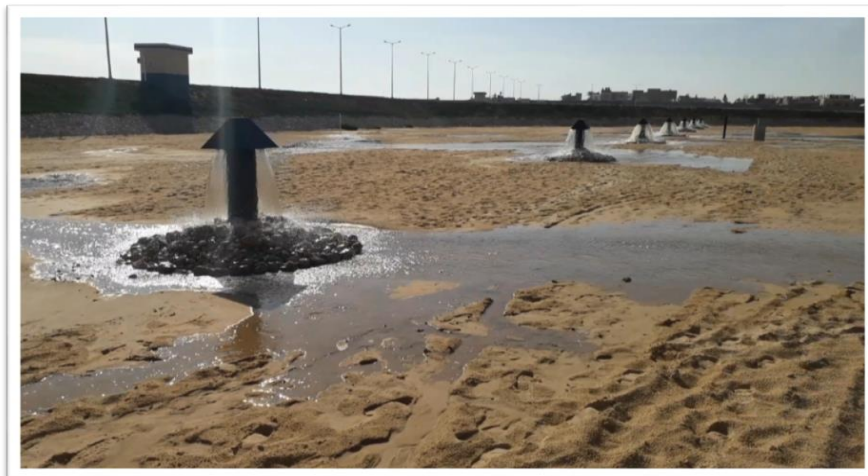
Figure 40 Infiltration Basin at Al Fokhari
