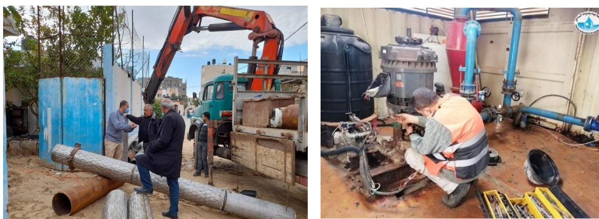
Figure 16 UNRWA water well-Khan Younis
