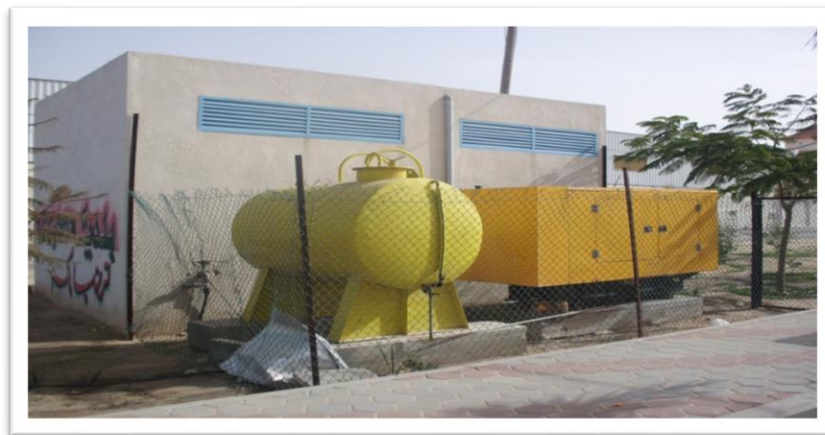
Fig (2) - 88 KVA generator in AlShokah on line booster station
