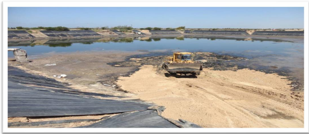
Fig (15) - KH Wastewater Treatment Plant
