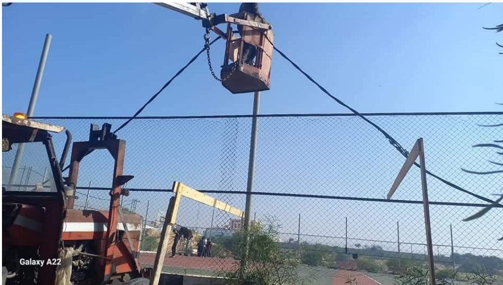
Operating Al Aqsa water well to serve more than 30,000 displaced people at Al Aqsa university
