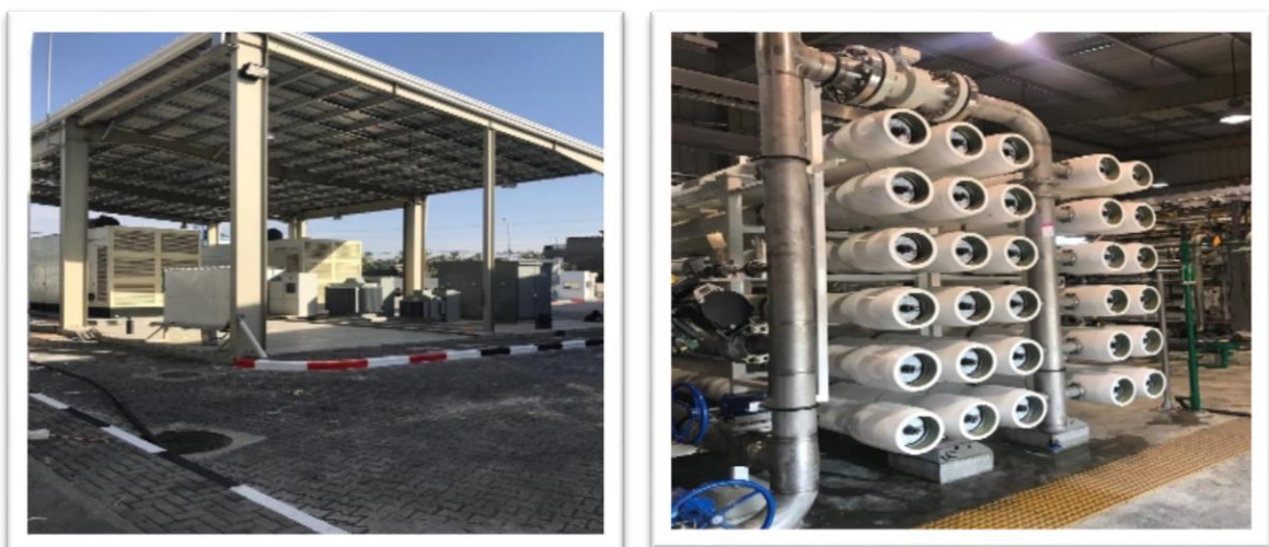
Figure 15: Deir Al Balah Sea Water Desalination Plant
