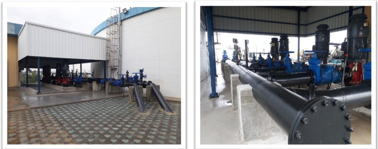
Figure 22: Al Rahma Booster station
