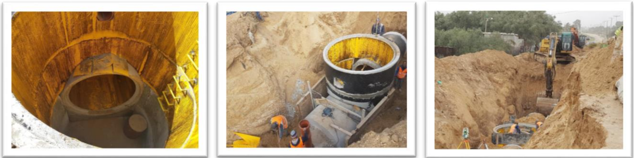
Figure 26: Central WWTP Gravity Pipeline
