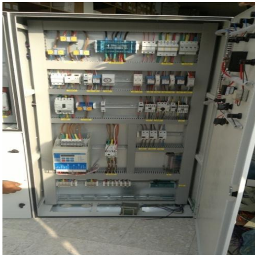
Figure. 15 Electrical Control Switch board
