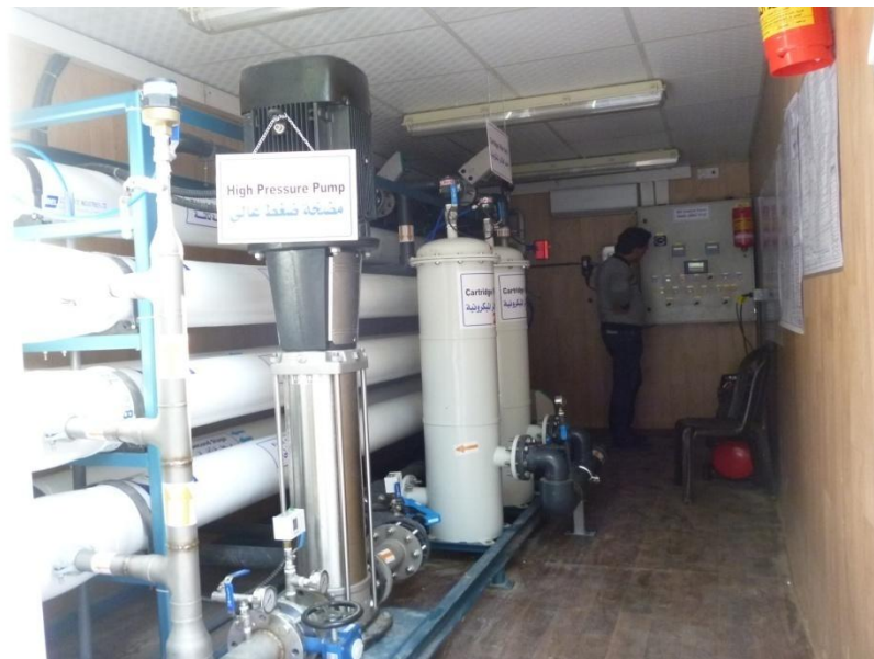
Figure 11. Taj Al Waqar Water Desalination Plant-Al Nussirate
