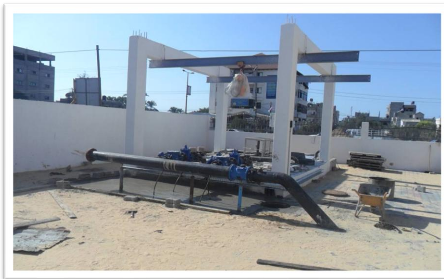
Figure. 23 Bani Suhaila Pumping Station
