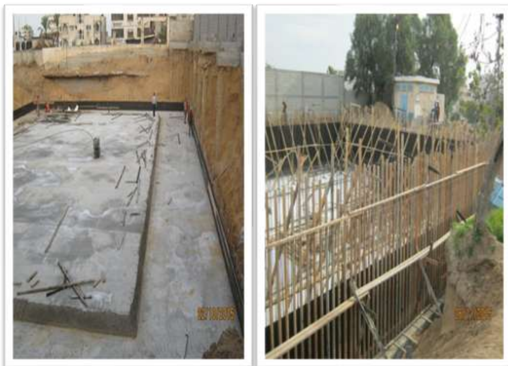
Figure 22: Al Sheikh Radwan Blending Tank
