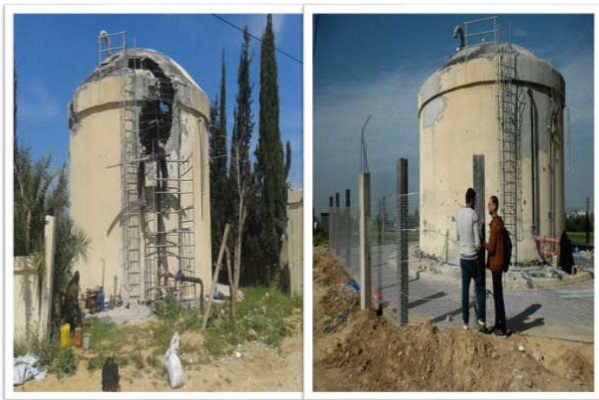
Figure 30: Al Musadar Water Tank
