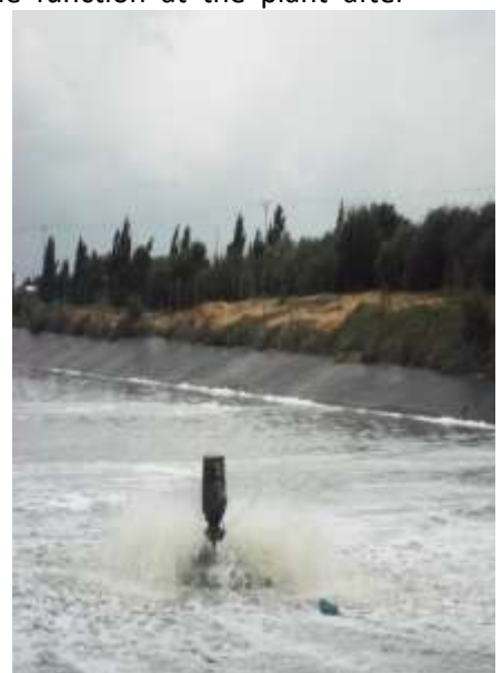
Figure 35: Beit Lahia Wastewater Treatment Plant
