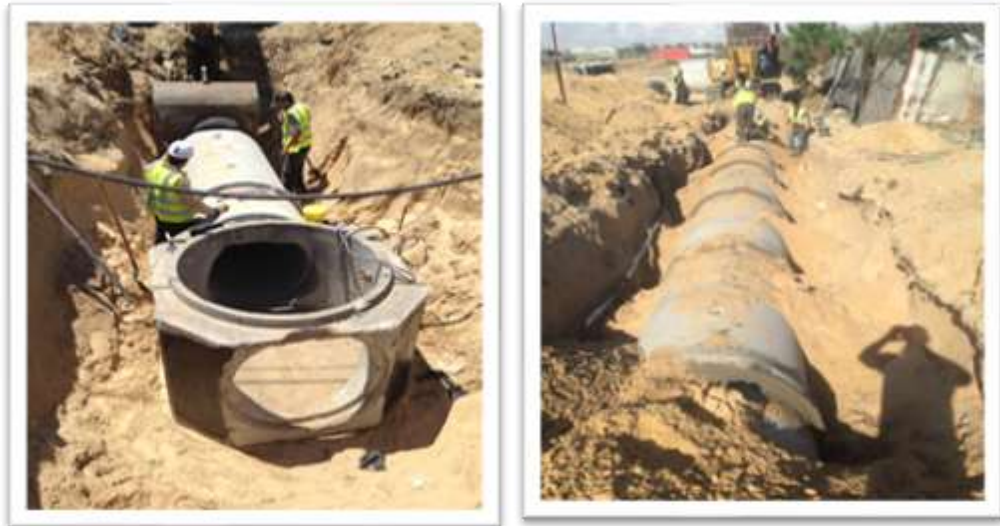
Figure 41: Abeda Storm water pipeline
