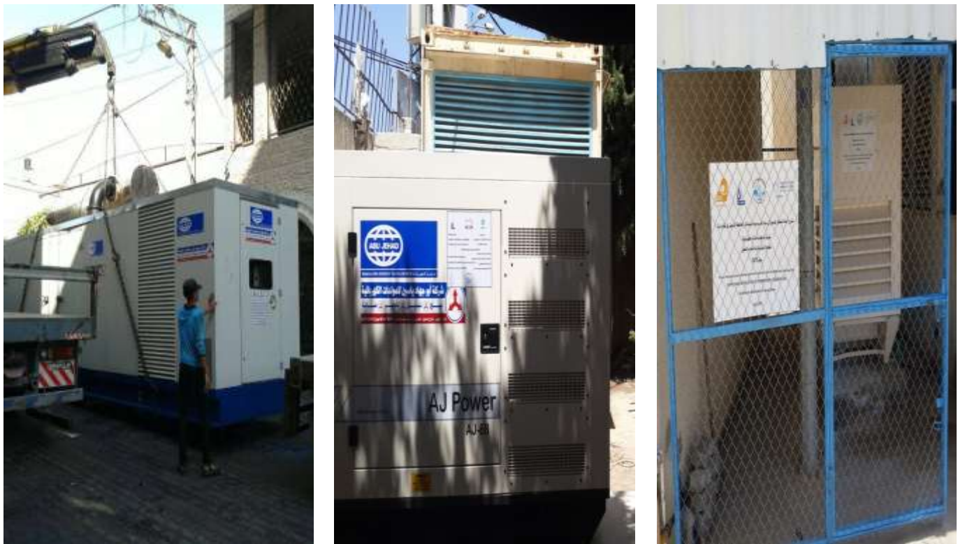
Figure 8 : Standby Generators Activities
