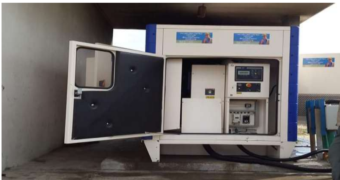
Figure 19: Filling the generator daily fuel tank with Diesel
