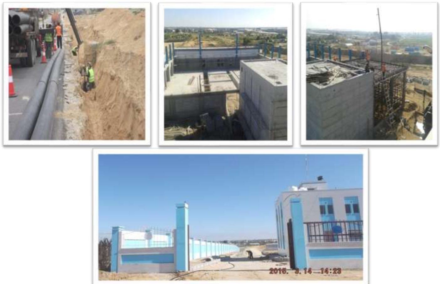
Figure 21: Sea Water Desalination Plant – Southern Governorates
