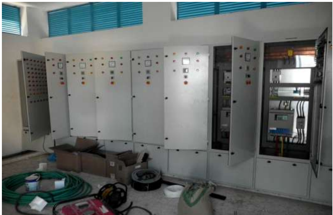
Figure 17: Electrical Control Switch board for Bani Suhail Water Tank Booster Station
